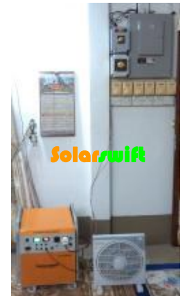
Model 2000W connecting With DB ( Grid/TNB & Solar System)
